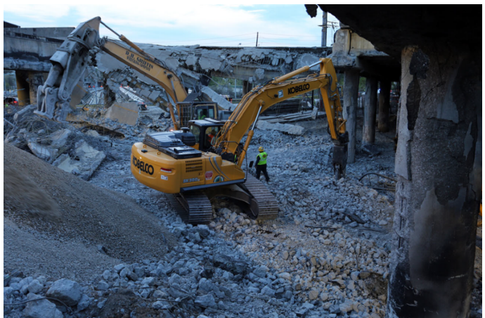
Figure 3: Post-fire damage at I-85 bridge in GA, USA in 2017. Collapsed girders and spalling of the concrete layer of the piers are visible (Kodur & Naser 2021b).
