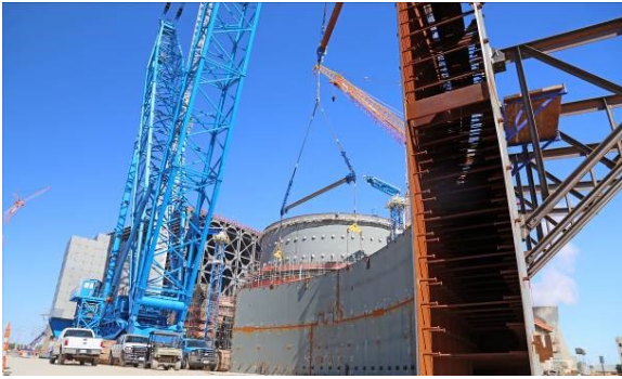
Figure 6: Lifting up of steel panels by the crane (Vogtle Plant Construction Photos).
