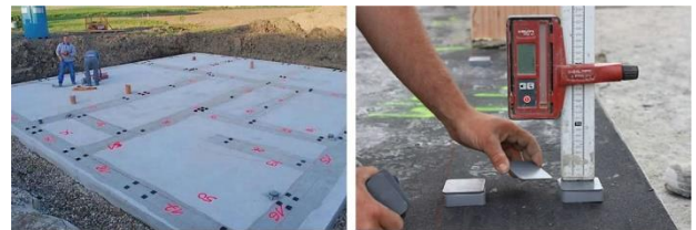
Figure 4: The preparation of construction site according to the assembly plan (Redbloccystems® ©2018, Redbloc®/Montageschritte ©n.d.)
