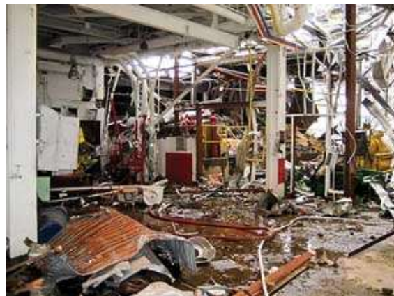
Figure 10: Damages made by hydrogen explosion at Muskingum River Power Plant's 585-MW coal-fired supercritical Unit 5. (Neville, 2009)
