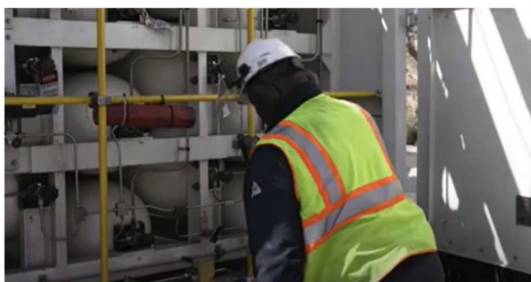
Figure 9: Picture of the tanks carried of the truck, checked after the burning seized. (Los Angeles County Fire Department, 2020)
